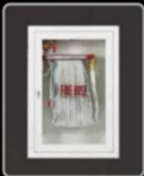
Fire Hose Cabinet
